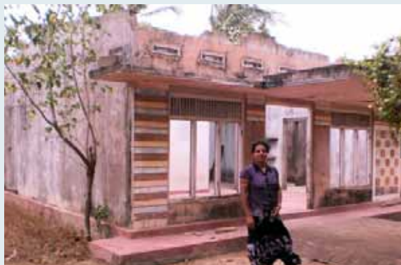
Mrs. K. Sivagowri's damaged house before the repairs. © P Jeyanthiran/UN-Habitat
