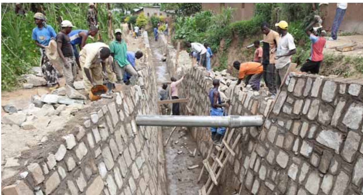
Construction of water drainage that is supported by UN-Habitat and ONE UN in Bugesera, Rwanda. © UN-Habitat /Julius Mwelu
